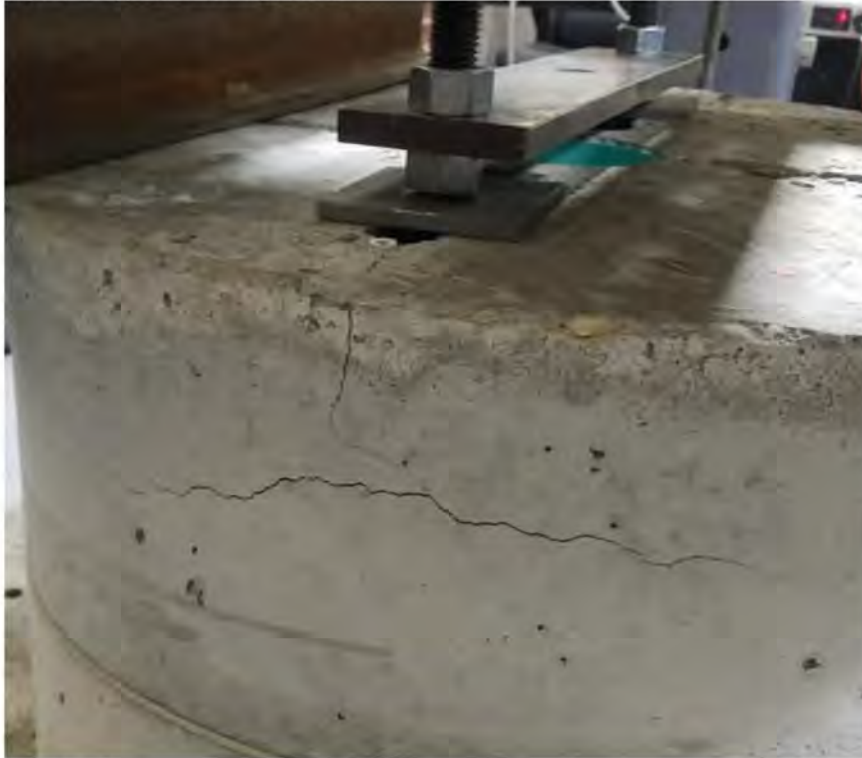
Figure 4: Typical Cracking Pattern
